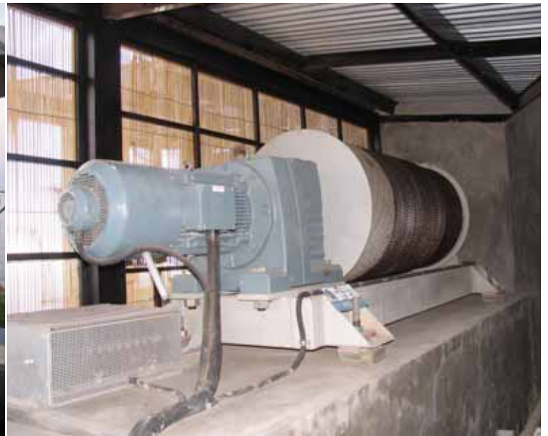
The machine room
